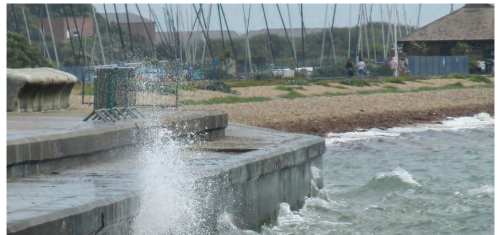
Wave overtopping at Stokes Bay
