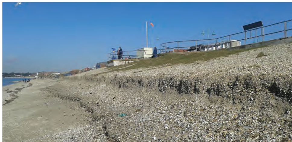
Beach erosion at Lee-on-the-Solent following a storm
