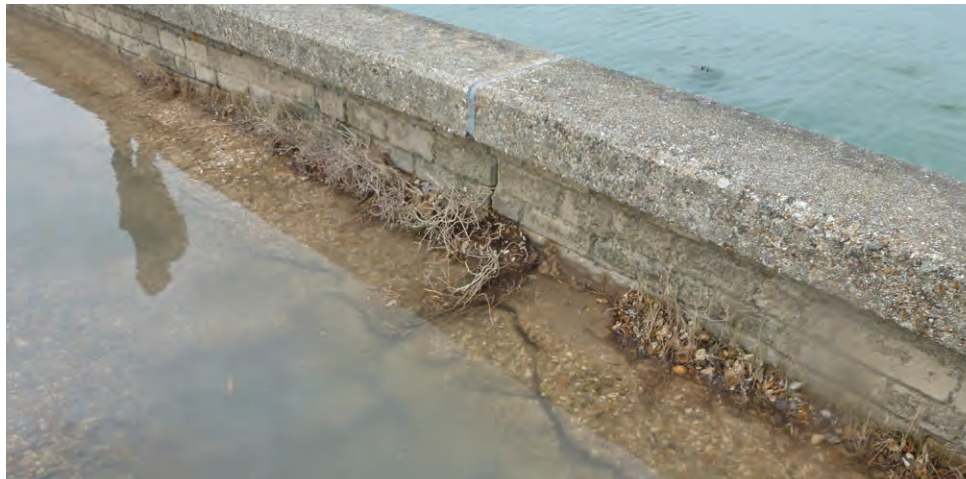
Sea wall at Hook Lake damaged by the winter 2013/2014 storms
